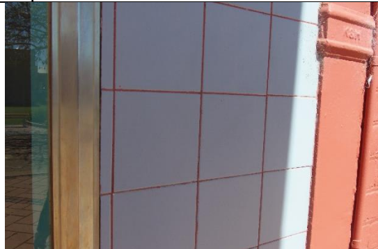
Tiles surrounding windows Source: Stephen Carrick Architects September 2021
