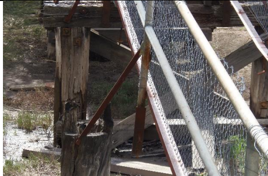
Damage to timber pillars Source: Stephen Carrick Architects October 2021
