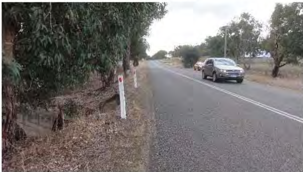
Finding 2.9 – Safety issues around culvert –Culvert within clear zone with no protection
