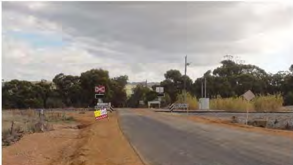
Finding 2.7 & 2.25 – Pavement markings missing removed from roadworks, and narrow approach seal 2.7 m – Also note singled sided speed zone
