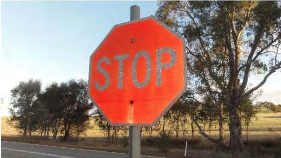
Finding 2.16 – Sign and warning device sign condition
