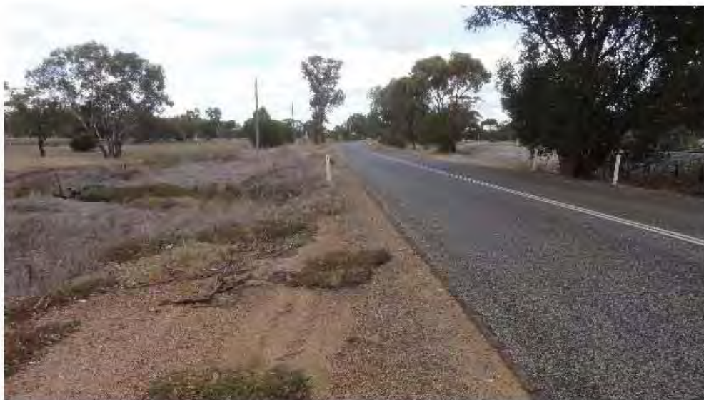
Finding 2.9 – Safety issues around culvert – Widened area prior to culvert
