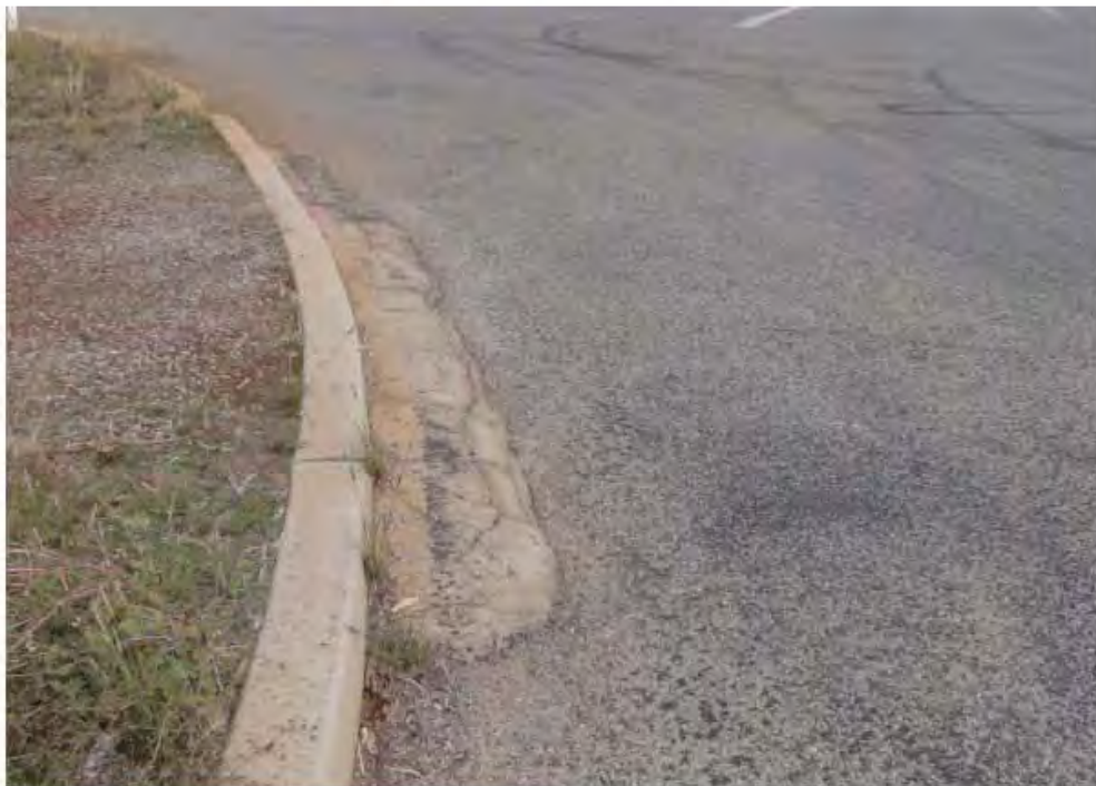
Finding 2.13 – Muresk Road intersection – Barrier kerbing used
