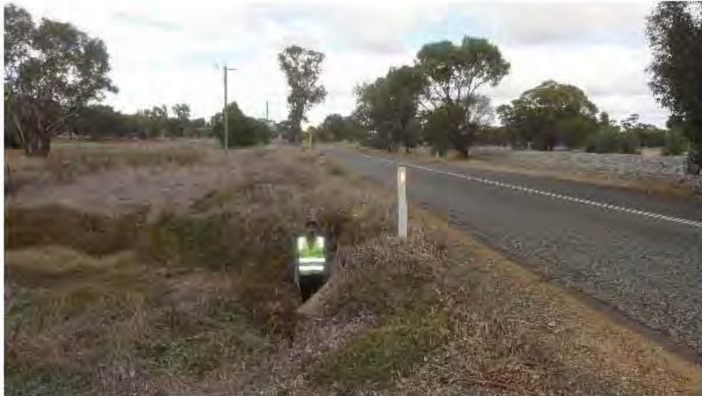
Finding 2.9 – Safety issues around culvert – Tall culvert within clear zone with no warning or protection other than a single guidepost (that is typical treatment of the road without culvert hazards)
