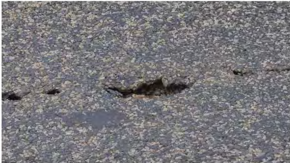
Finding 2.10 – Surface Condition – Example of road damage
