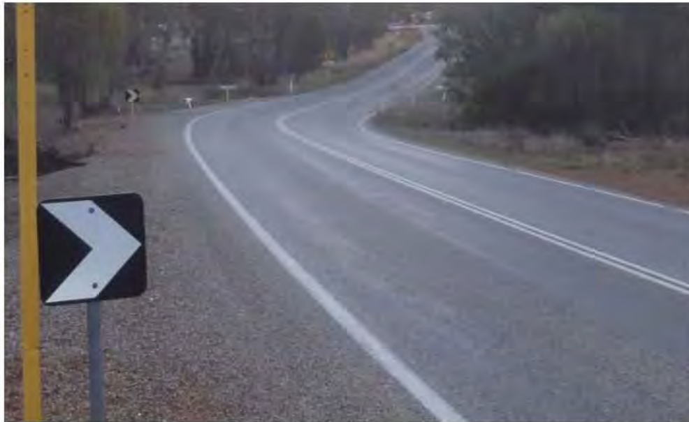
Finding 2.19 – Curved alignment markers – Incorrect and damaged signs present
