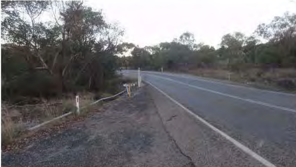
Finding 2.9 – Safety issues around culvert – Tall culvert within clear zone with no warning or protection
