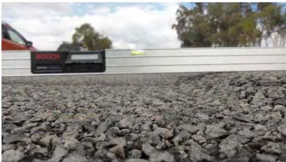
Finding 2.10 – Surface Condition – Road Deformation
