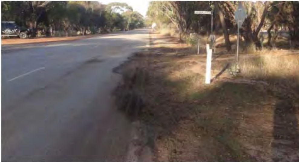
Finding 2.18 – Access Track – Debris on road
