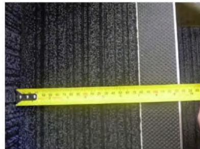
Nosings lacking contrast on stairs
