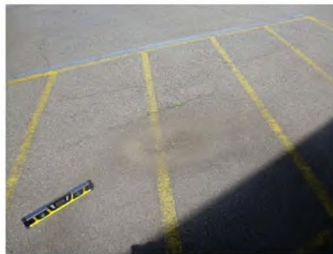
Uneven ground surface within shared area adjacent to Fitzgerald St
