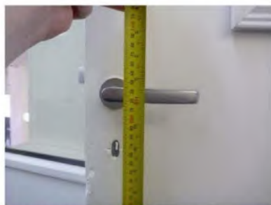
High door control (1230mm) at the Swan Room
