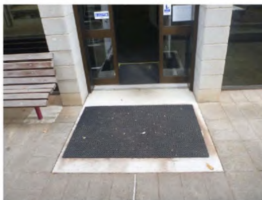
Mat creating a trip hazard to enter the Library
