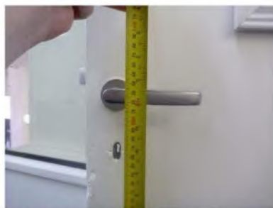
High door control (1230mm) at the Swan Room
