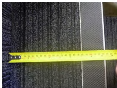
Nosings lacking contrast on stairs
