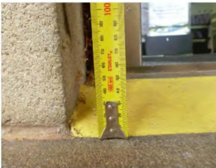
60mm abutment at threshold to enter the Library at the second entrance
