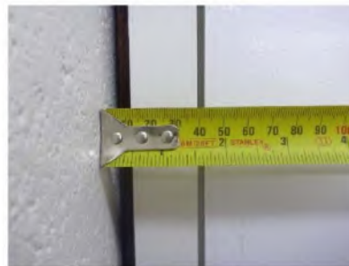
Reduced latch clearance (40mm) to exit the Swan Room
