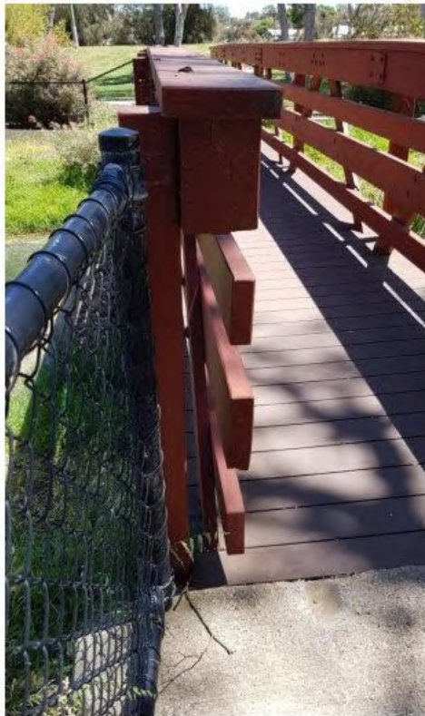
Photo 12: A significant hazard to cyclists.
