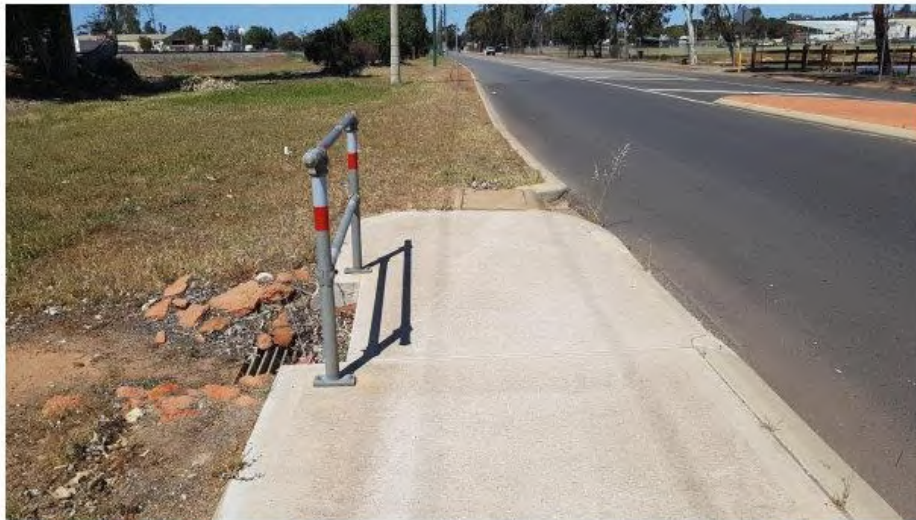
Photo 14: This barrier does not effectively protect road users from the grating, but does present a hazard.
