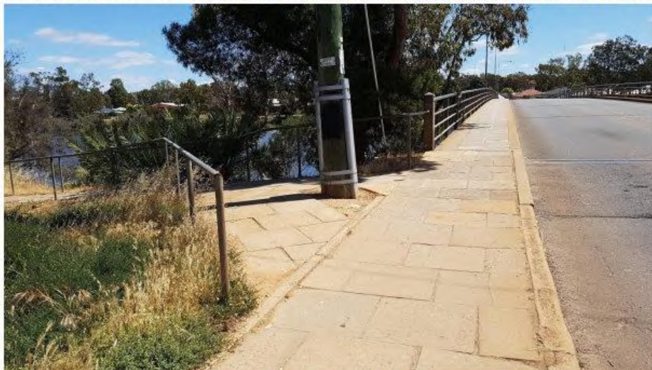
Photo 15: Poor barriers that could cause injury, especially to cyclists.
