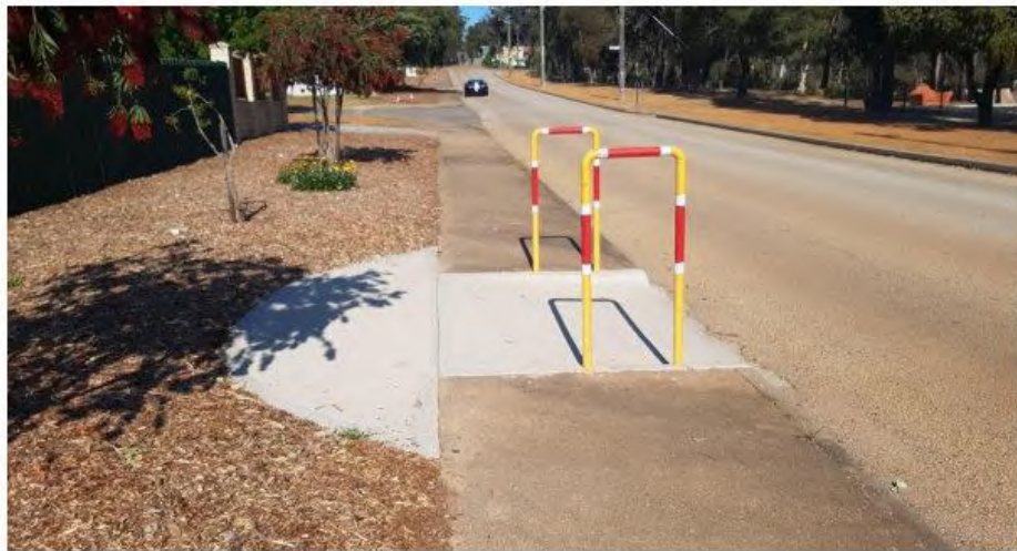
Photo 24: Not all cycling facilities are installed to standard.
