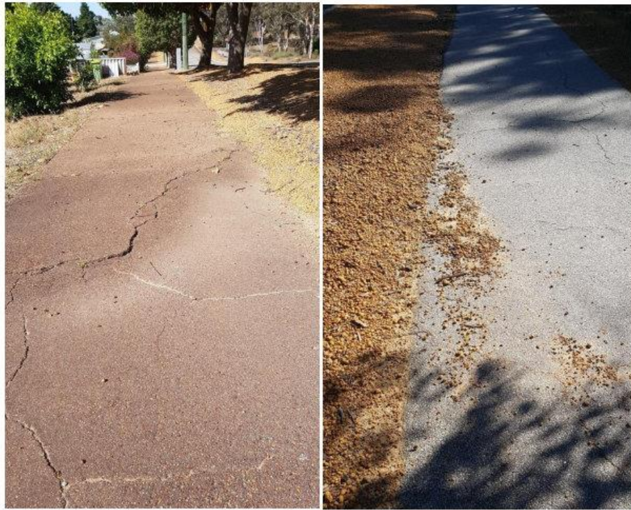
Photos 20 & 20a: Loose material and pavement defects along the path in Baker's Hill.
