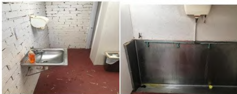
Figure : Current state of the men's public toilet.
