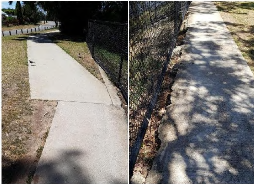
Photos 22 & 22a: Hazards to path users, and particularly cyclists.
