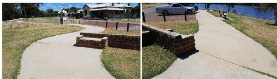
Photo 19: This handy stone bench presents a significant hazard to path users.
