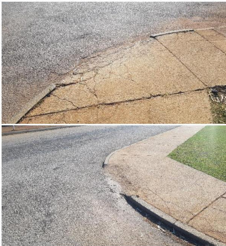
Photos 13 & 13a: These examples of sub-standard pedestrian ramps are in Wundowie.
