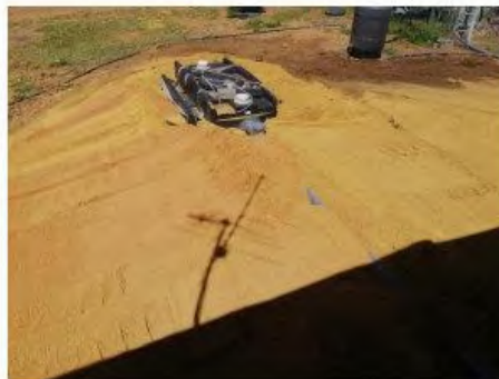
Septic tank showing painted pipes
