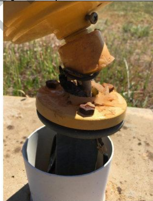
Image 8: Broken Light Fitting
