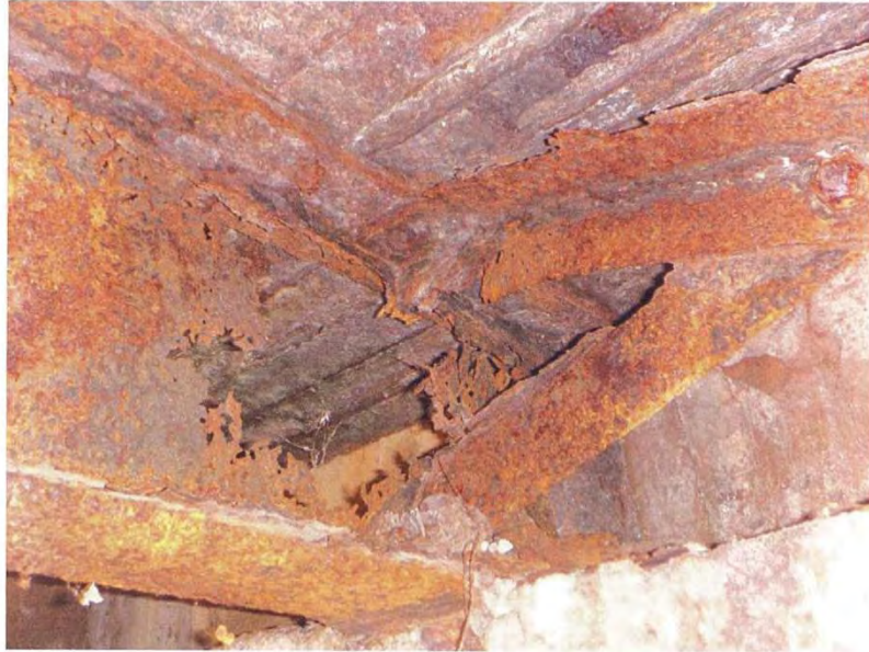
Photograph 7: Corrosion perforation to Abutment 1 end of Beam 9.
