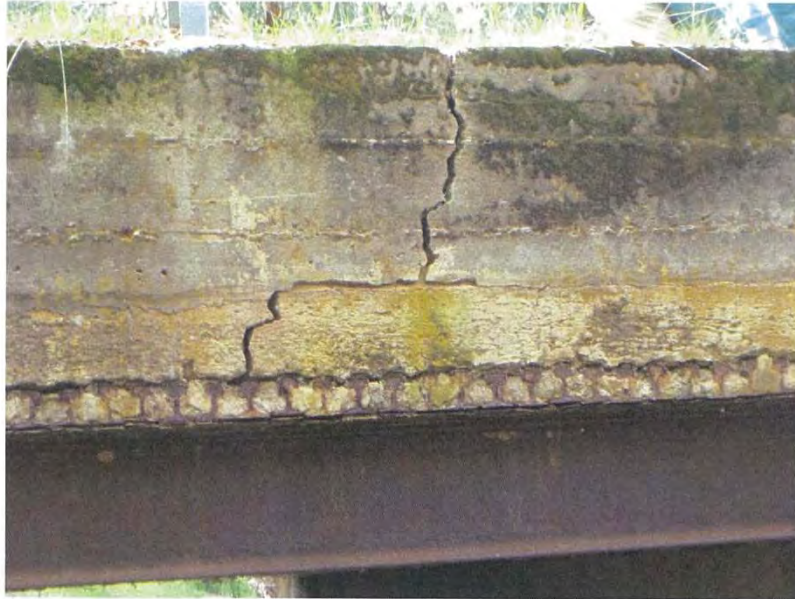
Photograph 11: Crack to concrete deck edge.
