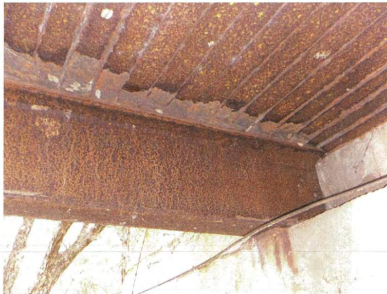
Photograph 10: Typical corrosion to beams and transverse beams.
