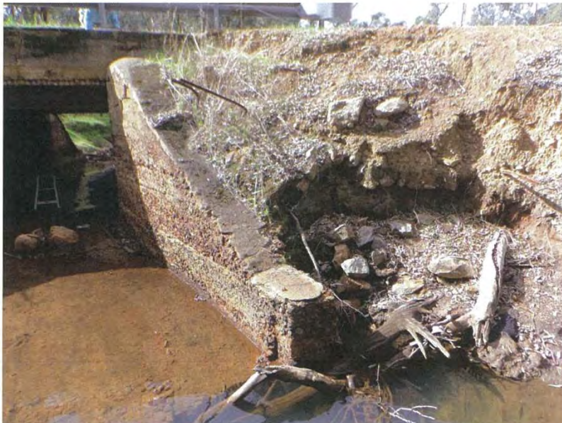
Photograph 14: Scour behind Abutment 1 Left Hand Side Wing Wall.
