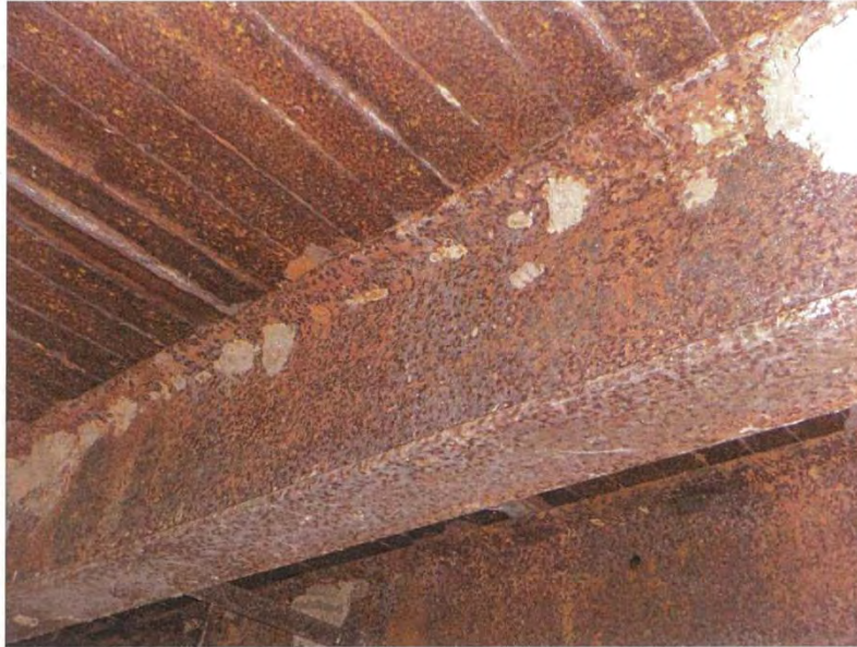
Photograph 9: Typical corrosion to beams and transverse beams.
