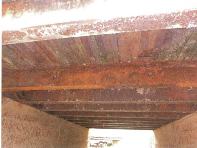
Photograph 5: Underside of bridge – note widespread corrosion to beams.
