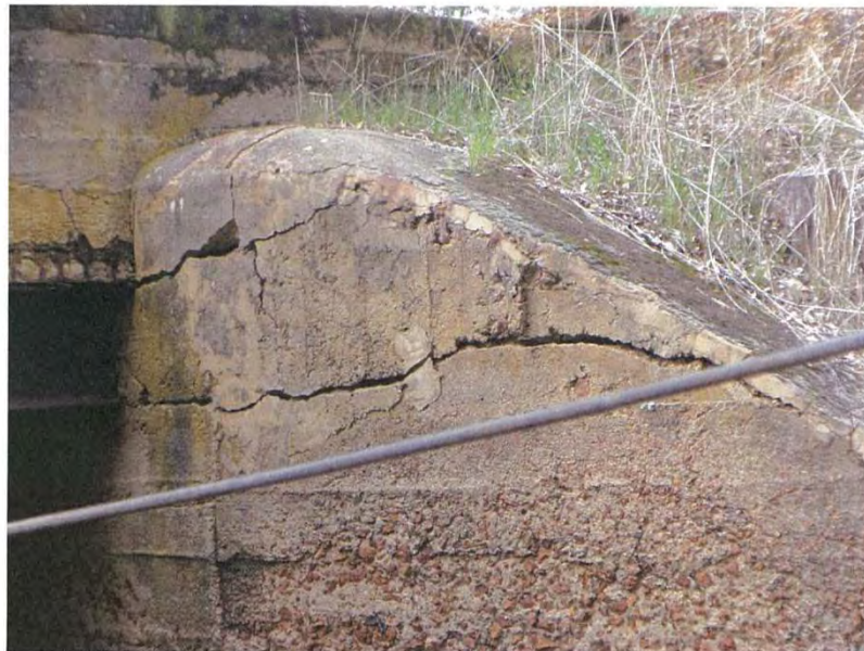
Photograph 12: Cracking to Abutment 1 Left Hand Side Wing Wall.
