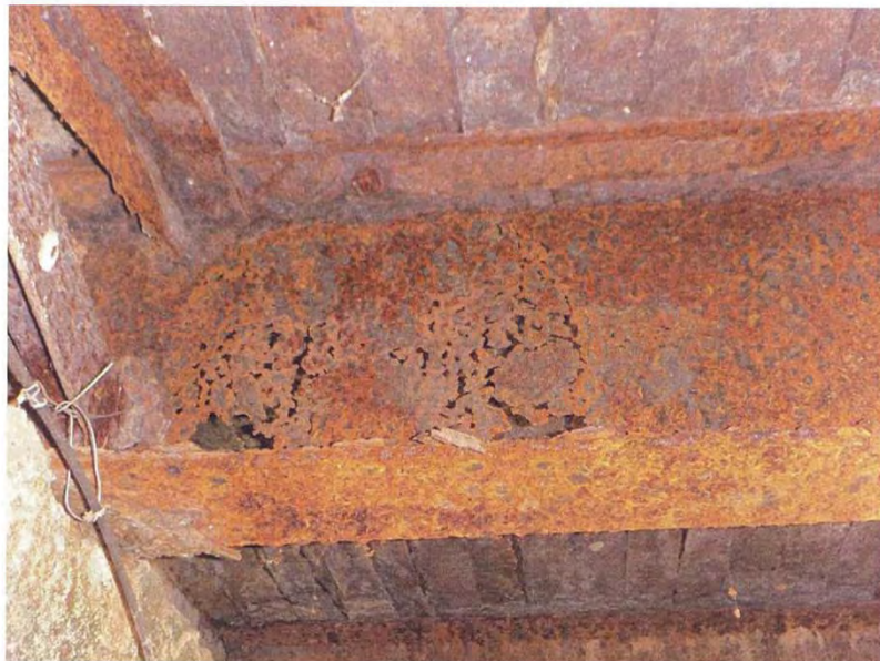
Photograph 8: Corrosion perforation to Abutment 2 end of Beam 9.
