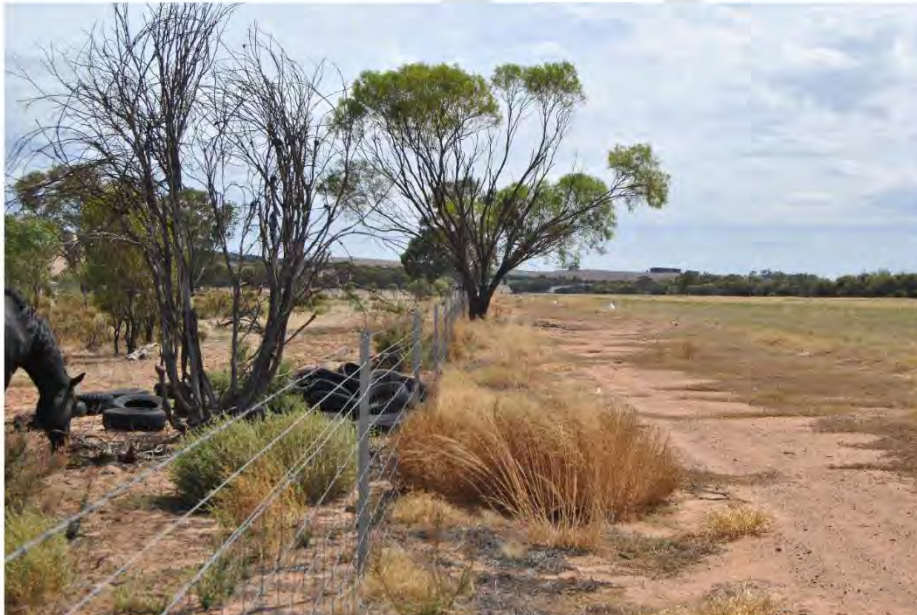
View facing north-west along the airport perimeter fence. The runway strip edge cones can be seen. Trees may infringe the transitional surface and should be assessed by survey to ensure the flyover areas are clear.
