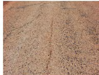
Existing issues: Surface Age
